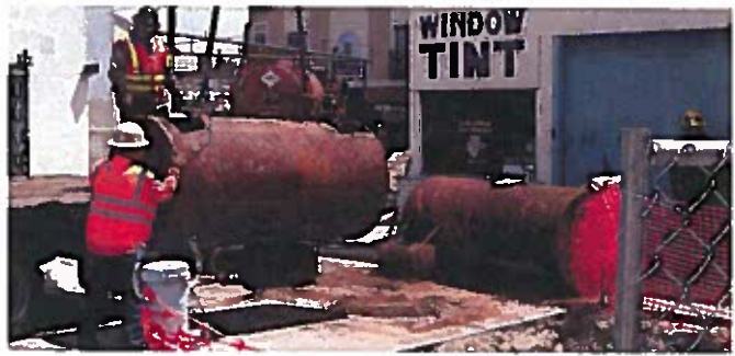
A fueling and service station, closed in the 1970s, is assessed before being redeveloped into a new restaurant and affordable housing complex in downtown Bellflower.
